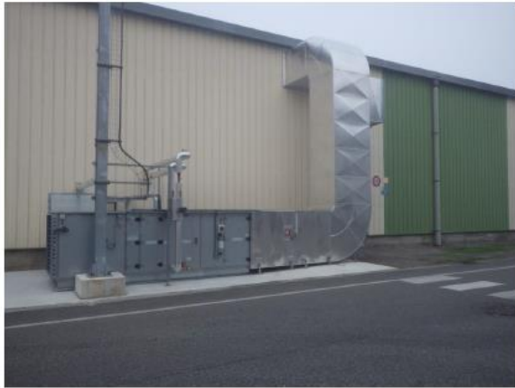
Chauffage hangar Dermulsène
