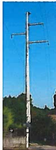
Exemple d'un support béton monopodes (type K2F).
