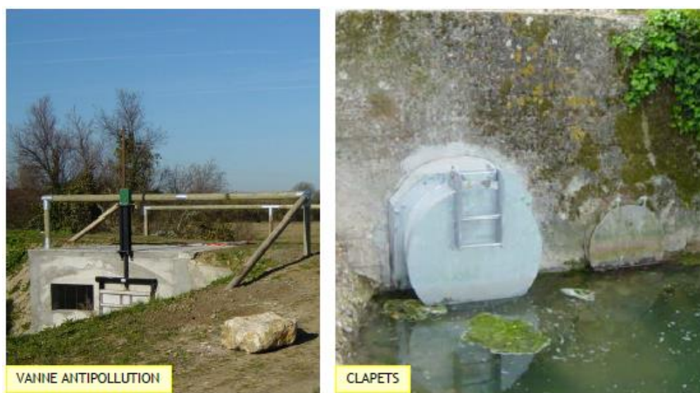
Figure 6: Dispositif anti-pollution "Vanne-clapet des Sartières"
